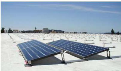
USF, 500kW roof-mounted
