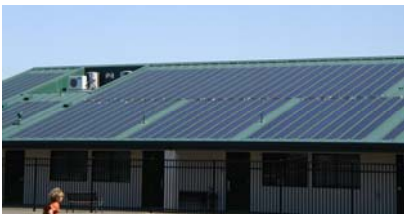
Greenbrook School, 130KW PV System
